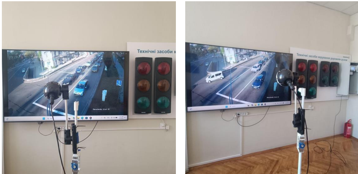
Figure 2. Installing and configuring the video detector FLIR TrafiCam 4TI ETH
